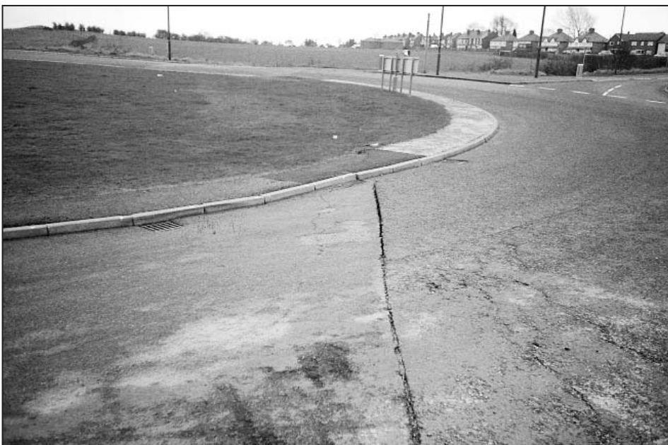
Figure 8. The latest in a series of fault reactivation phases, from 1991 to 2000, causing moderate to severe damage to the A610 bypass at Ripley.
