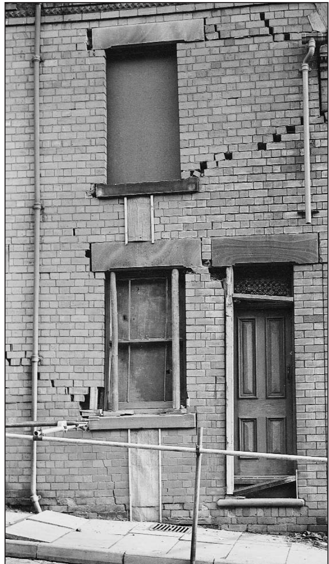
Figure 7. Damage to a terraced house in Belvoir Street, Hucknall, in 1955. The house has since been rebuilt.
