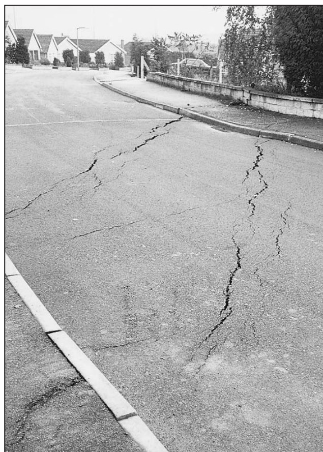
Figure 3. Reactivation of the Inkersall Fault in the 1980s, caused widespread damage at the northern end of the Inkersall Green housing estate; this small graben feature formed across a road over a subsidiary fault within the Inkersall fault zone.
