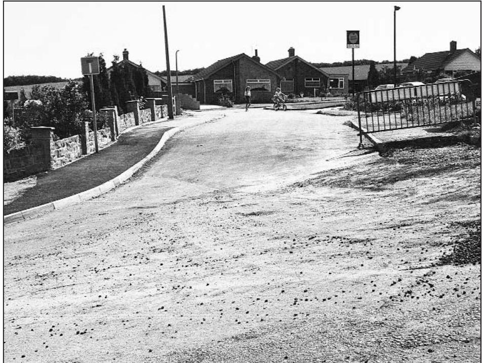
Figure 9. A fault scarp across a road in a housing estate at Inkersall, near Chesterfield, has reactivated as successive coal seams have been mined from beneath, causing repeated damage to the road and adjacent houses.
